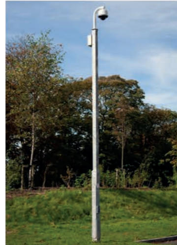
Tilt Over - Square CCTV Columns (TPS)
