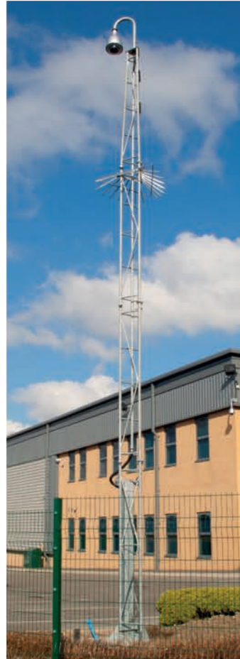
Lattice Towers (WDT)
